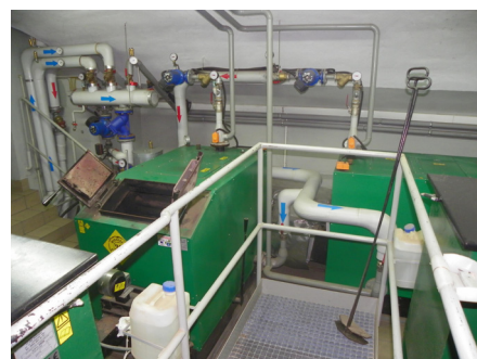
The co-financed installations for the incineration of biomass (wood pellets) with a total capacity of 240 kW used for heating purpose in Primary school in Jordanów
